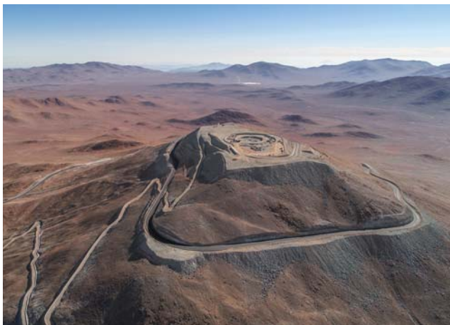
▲ FUTURE ELT SITE Taken in early 2018, this image shows the early foundations for the dome and telescope structure of ESO's Extremely Large Telescope (ELT), which will perch at an altitude of some 2,500 meters (8,300 feet) on Cerro Armazones in the Chilean Atacama Desert.
